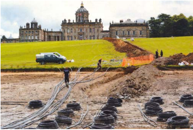
Installation of the Heat Recovery System Photo Courtesy of Ecovision Systems Ltd
