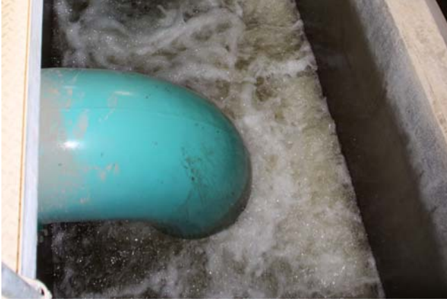
Discharge From One of the First Intake Pipes
