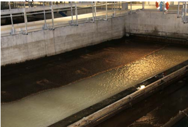
Dissolved Air Flotation Floc being skimmed off the COCODAF tank
