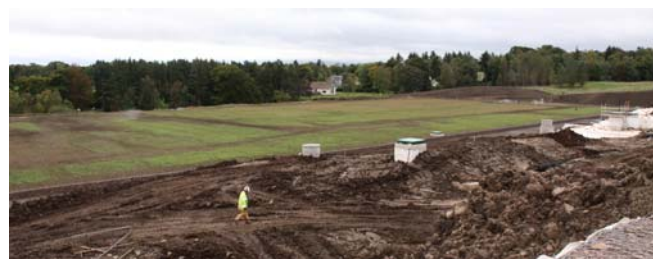
The Grass Cover to the Huge Clear Water Storage Tank
